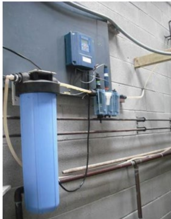
Figure 4: Chlorine and pH Monitoring System
