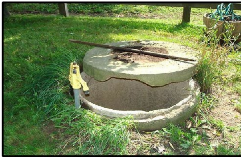
Figure 1: Damaged Lid and Casing
